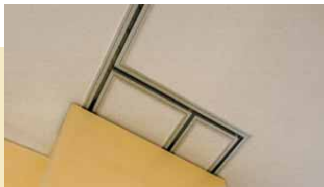
Particolare guide area impacchettamento Detail of the guide rail in the storage area
